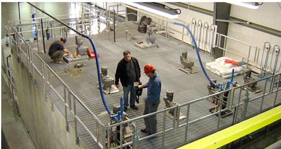
Two 4,000 m 3 /d concrete ACTIFLO® high-rate clarifiers successfully treat tailings water effluent, lowering arsenic levels in the discharge tailings water down to 0.02 ppm, well below Goldcorp's target. The plant's permitted limit for arsenic is currently 0.25 ppm.
