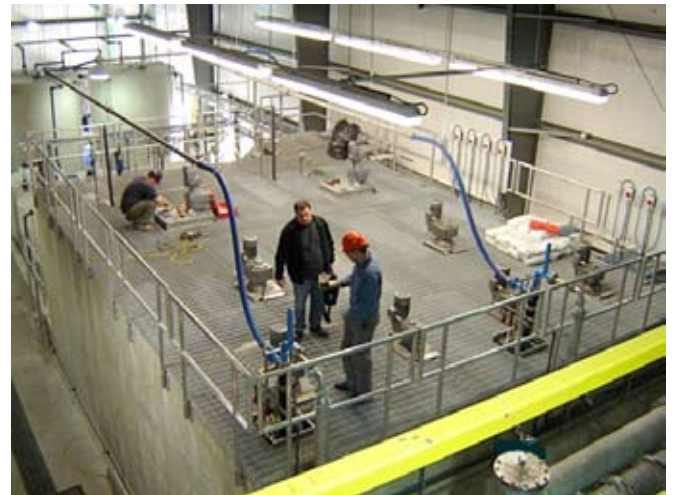
Two 4,000 m 3 /d concrete ACTIFLO® high-rate clarifiers successfully treat tailings water effluent.
