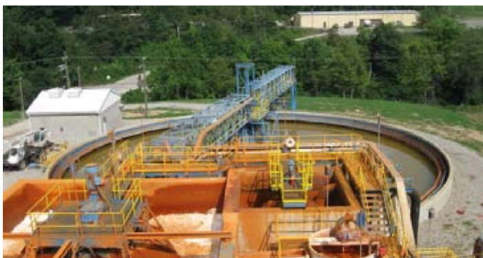
Water is pumped from mine pools to lower the water level to an elevation below the Sewickley seam, then treated prior to discharge.
